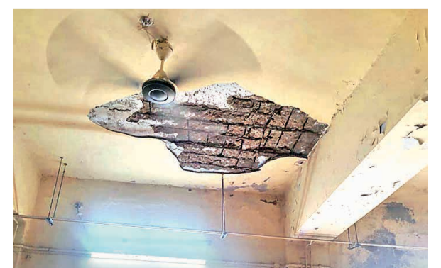
A portion of the ceiling fell in Jawaharlal Nehru Medical College (JLN) Hospital's Male Medical 3 ward on Friday.
